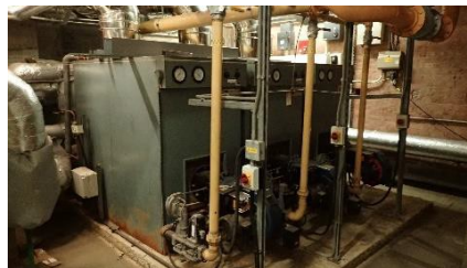
Figure 14: Decommissioned boiler plant.
