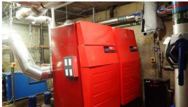
Figure 76: Robin Brook gas boiler plant.
