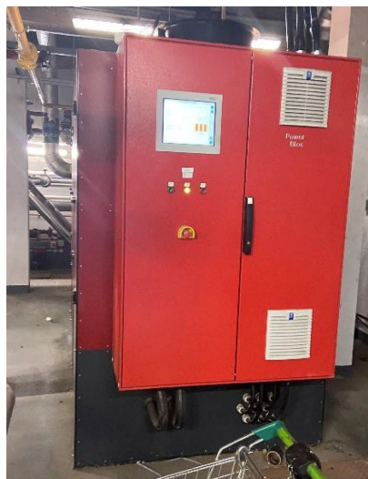
Figure 37: Combine Heat and Power (CHP) Pack.
