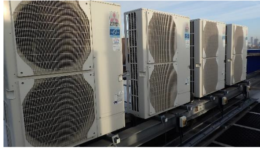
Figure 27: Existing roof mounted VRF
