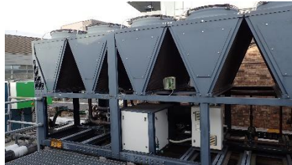
Figure 15: Roof mounted chiller.
