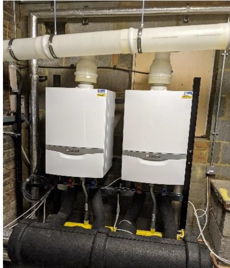
Figure 24: Newly installed boilers.
