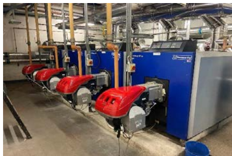
Figure 22: Main boiler plant.
