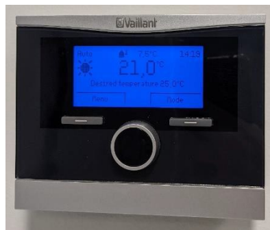
Figure 30: Note set-point of 25°C.
