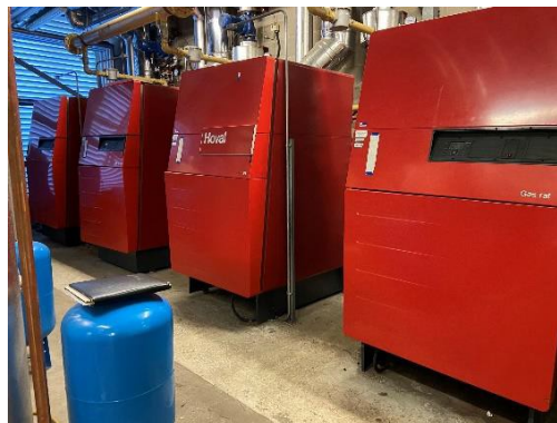
Figure 12: Main boiler plant.
