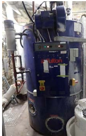
Figure 44: Steam Boiler Plant.
