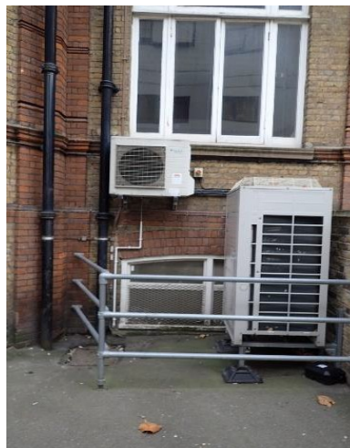
Figure 48: Ground Mounted VRF
