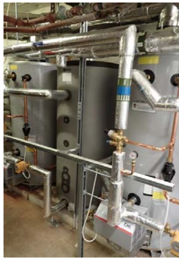
Figure 52: New DHW Calorifiers.
