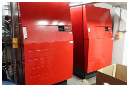
Figure 19: Phase 2 boiler plant.
