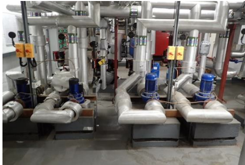
Figure 18: Main boiler house pump sets.
